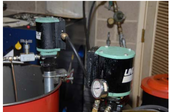
Testing PMV pumps in the St. Louis lab
