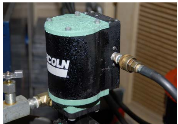
An even wetter oil pump on the same day
