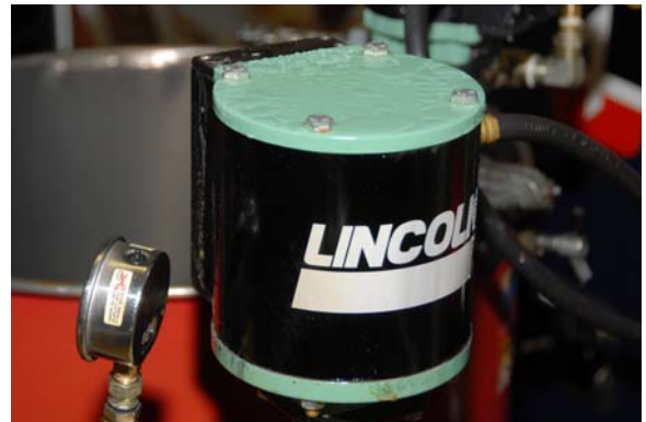
Water condensing on PMV grease pump on a hot, humid St. Louis Summer day
